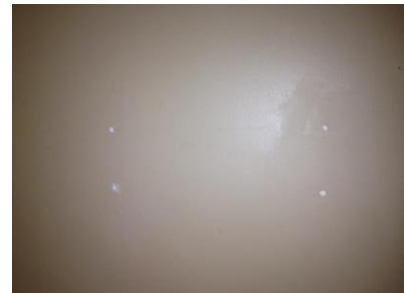
Holes Patched But Not Painted
