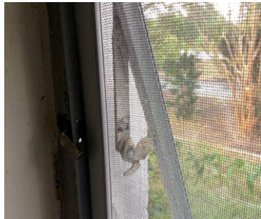
Broken Window Latches
