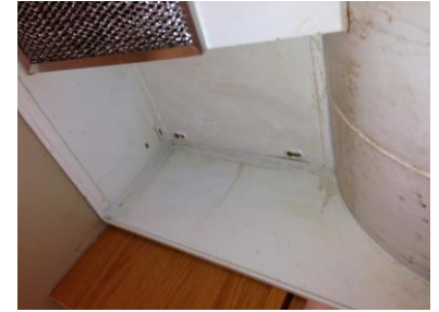
Hood Vent Greasy/Dirty
