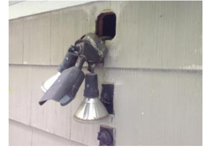
Broken Exterior Light Fixtures
