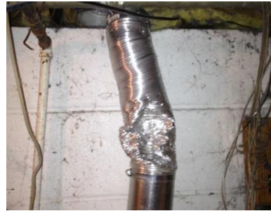
Dryer Venting Not to Code
