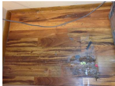
Behind Appliances Not Clean
