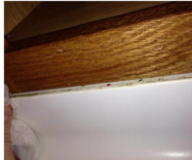
Grease/Grime on Cooking Surfaces
