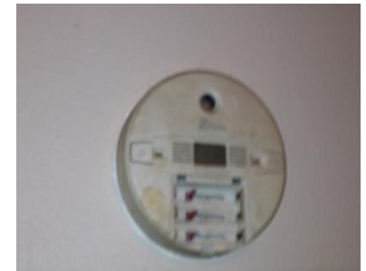
Batteries Missing from Smoke Detector
