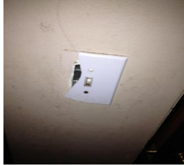
Cracked Switch Plates
