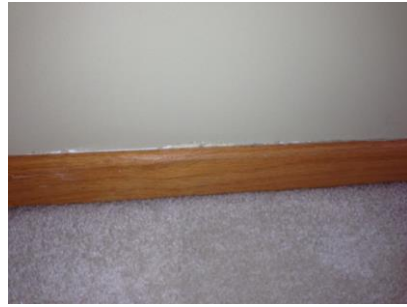
Dirt/Grime on Baseboards
